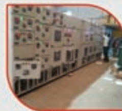
Power Room Termination
