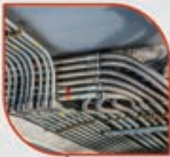
General Conduiting and Wiring
