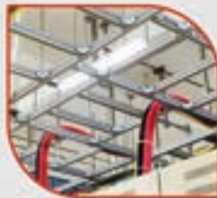
Cable Trays and Ladders
