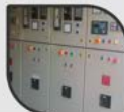
Synchronizing & Load Sharing Panels
