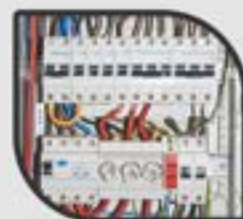
Distribution Boards -DBS
