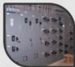
Motor Control Center -MCC
