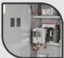
Auto Transfer Switch - ATS
